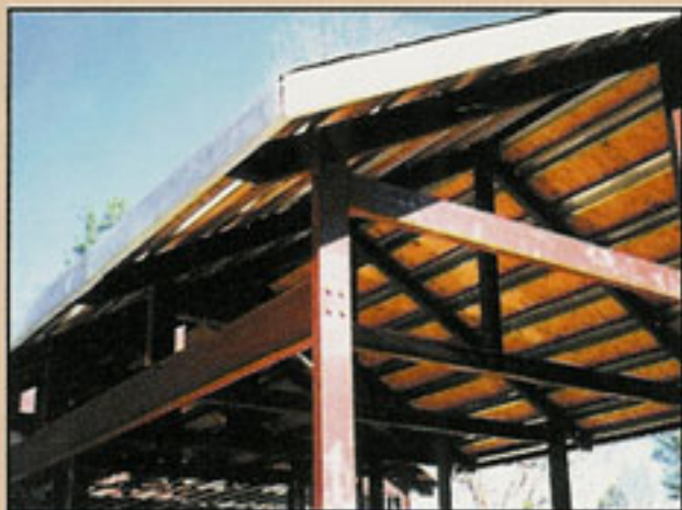
The roof is installed on the load bearing, "red iron" frames leaving wall, floor and ceiling construction in the "dry."
